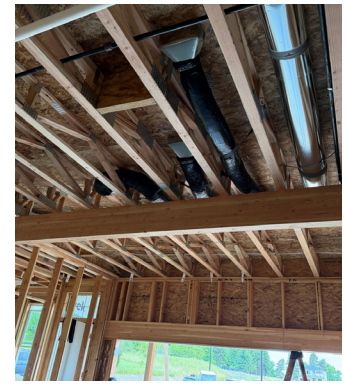
BEFORE: Visible ductwork can be seen underneath the subfloor of a front room before insulation is installed.
