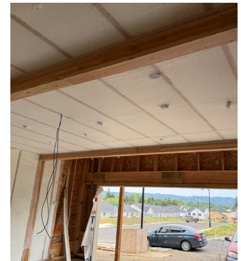
AFTER: Blow-in insulation is added to completely fill in the cavities beneath the subfloor of a front room to prevent gaps.
